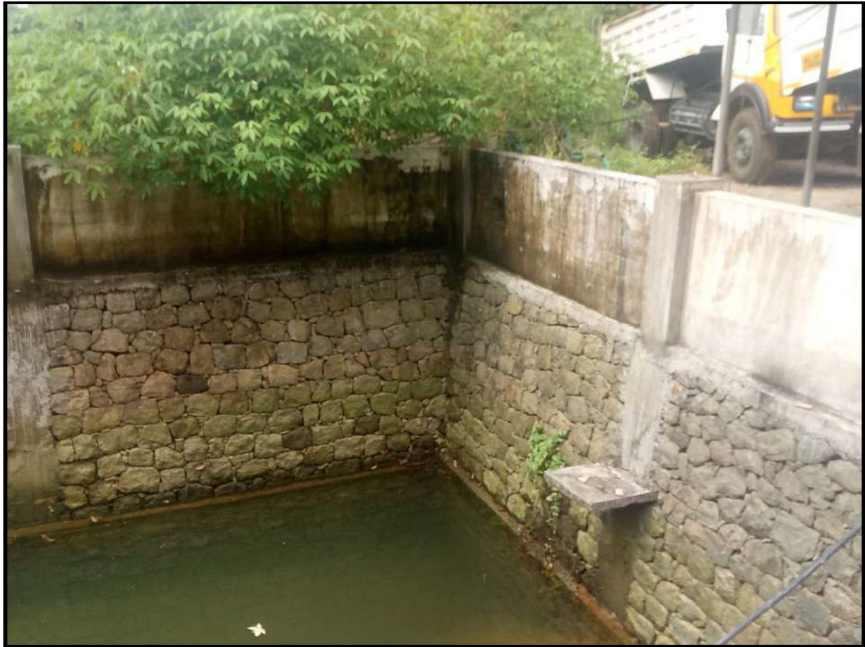
Photograph showing the rain water harvesting tank
